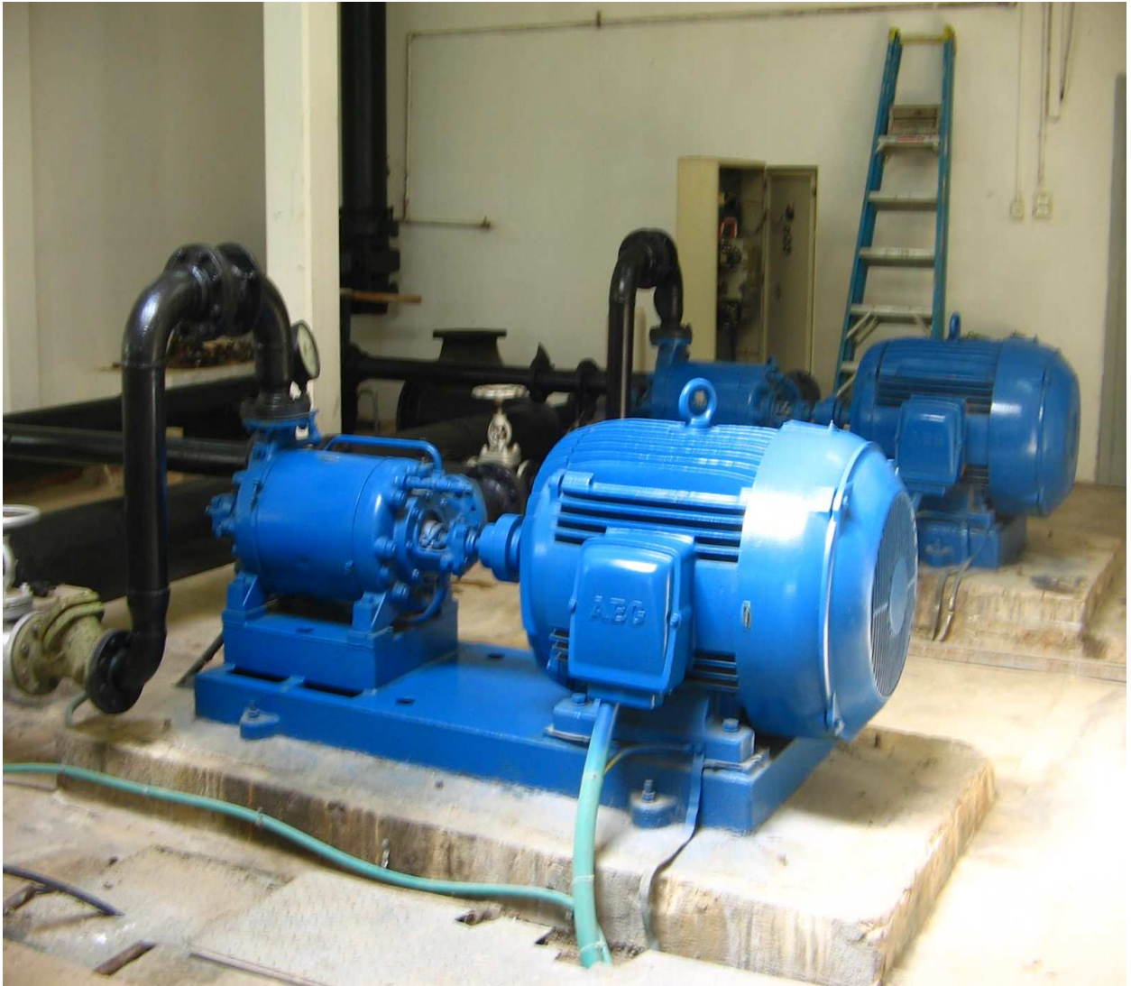
Appendix 5.4: Pumps in series that pump the water to the distribution systems
