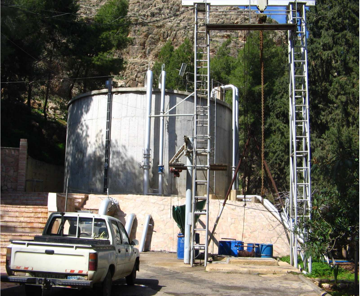
Appendix 5.2: Balancing tank which the ground water pumped to with 500 m 3 capacity.
