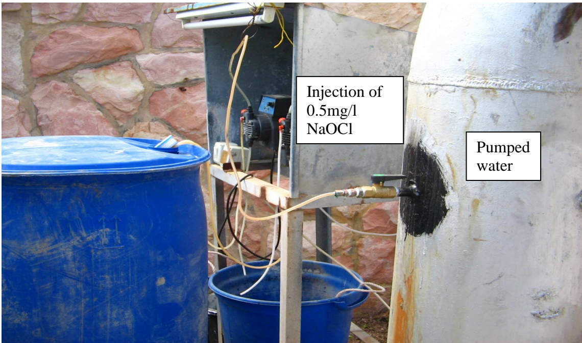
Appendix 5.3: Dosing pump which injected the chlorine to the pumped water to the distribution system
